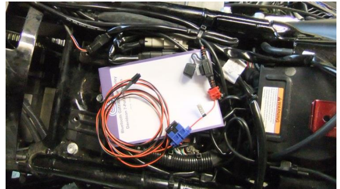
Connect 12V switched main supply
